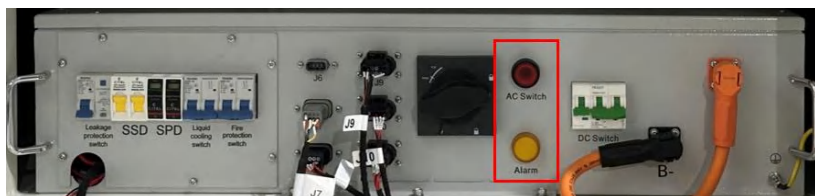
Fig 9-3High Voltage Box Indicator
